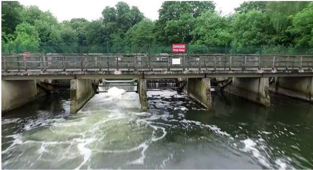
Berkshire Weir, River Thames, June 26, 2020, 2 fatalities
